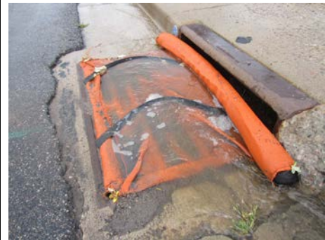
Inlets can be protected with filter fabric and filter socks, which trap sediment and allow water to flow through.
