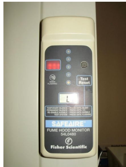
Fume Hood Monitor (Figure 4)
