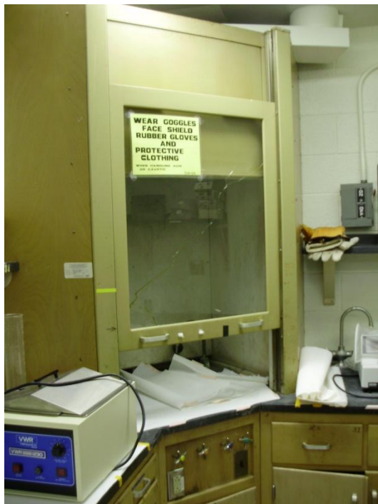
Room 272 Hood (Figure 5)
