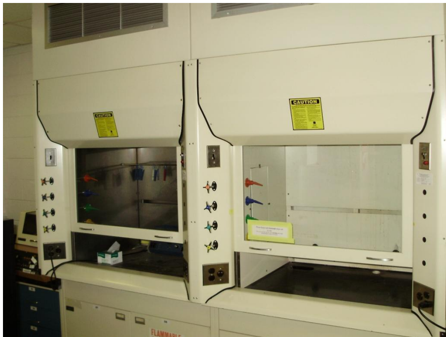
Room 159 Hoods (Figure 5)
