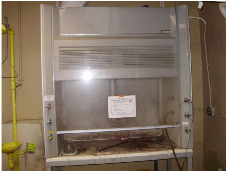
Room 120 Fume Hood (Figure 3)
