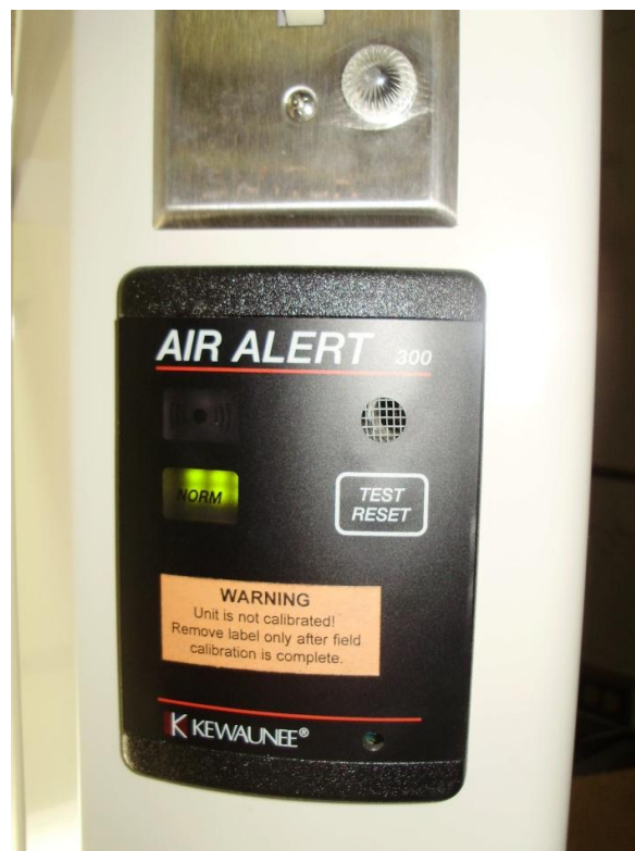
Fume Hood Alarm (Figure 6)
