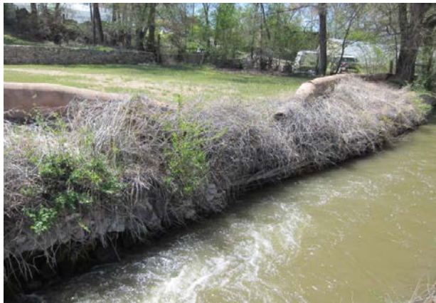
Figure 9 – Eroded Fence and Canal Wall
