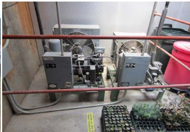
Figure 6 - Compressors need replaced.
