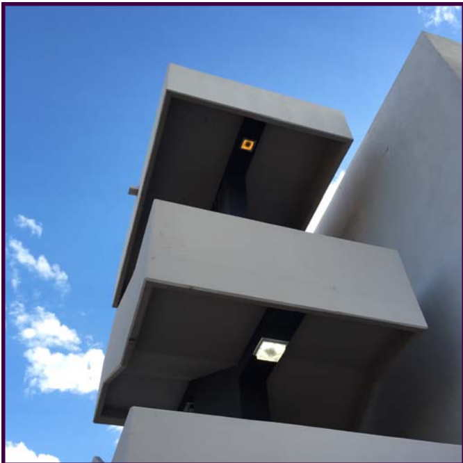
Old (top) and new LED (bottom) exterior light fixtures
