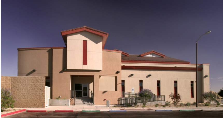
Satellite Chilled Water Plant
