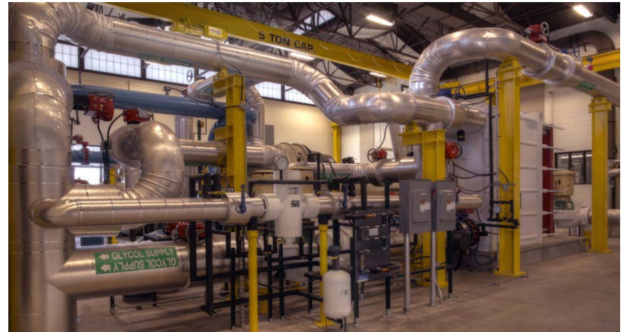
Satellite Chilled Water Plant Piping
